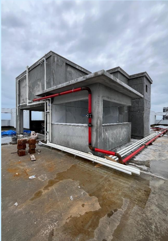
T1 TERRACE PLUMBING&FIRE
