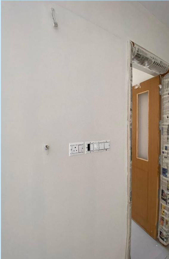
T2 7 TH SWITCH BOX FIXING
